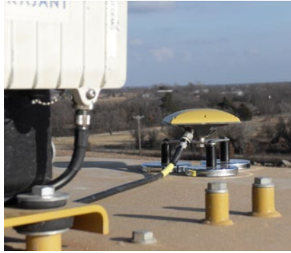
Roof mounted GPS antenna—fitted using high strength magnetic mount
